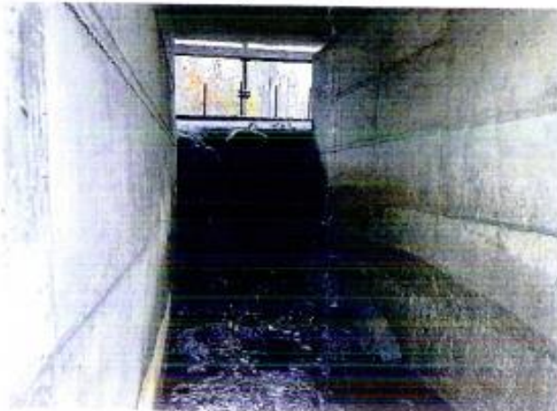
G - Debris in Spillway
